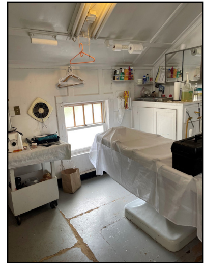
Figure 5 – Preparation room with a floor that didn't appear to be impervious.
